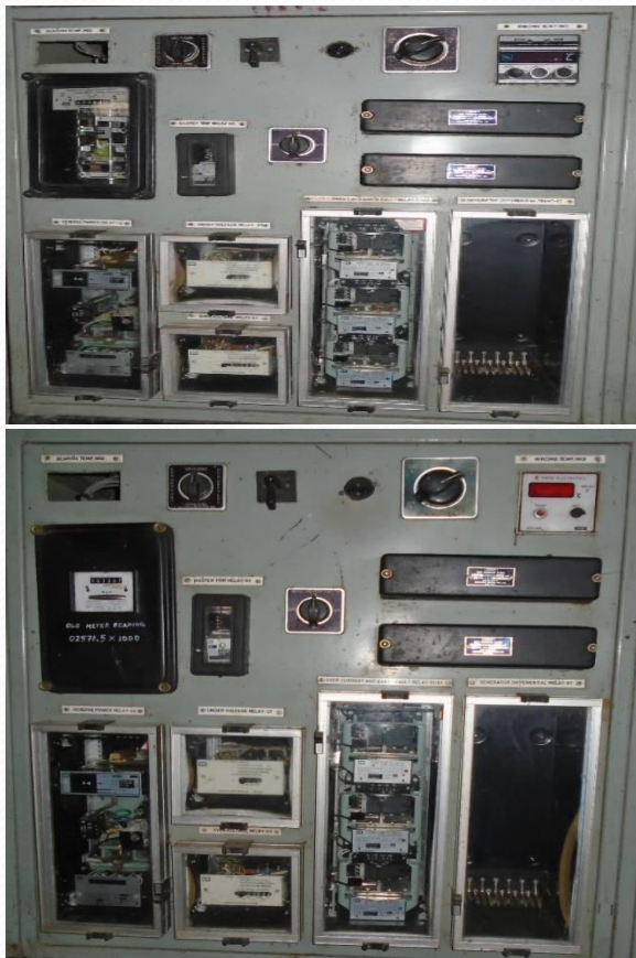
OLD INDOOR CONTROL UNIT PANELS
