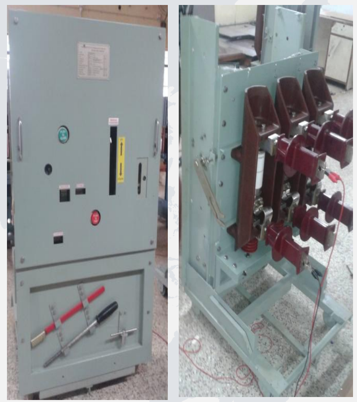
S&S – VCB (HHV12)
