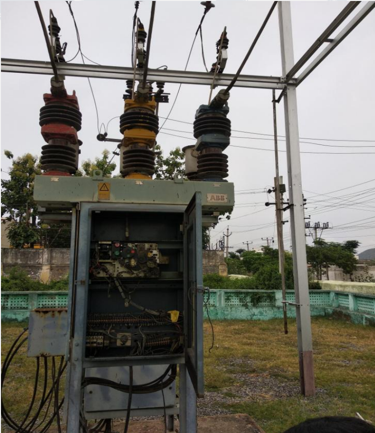
ABB-OUTDOOR BREAKER (1250A,25kA)
