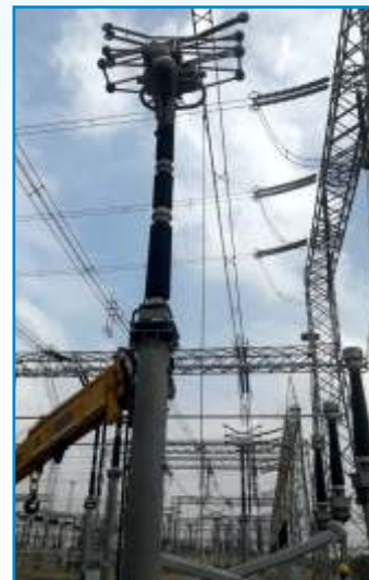
Other Make Disconnector (Before Retrofit)
