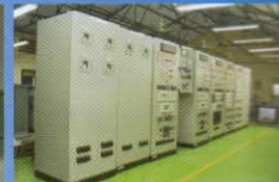
Control & Relay Panel
